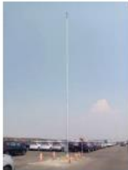
PT PBW Crushing Samarinda LPS External
